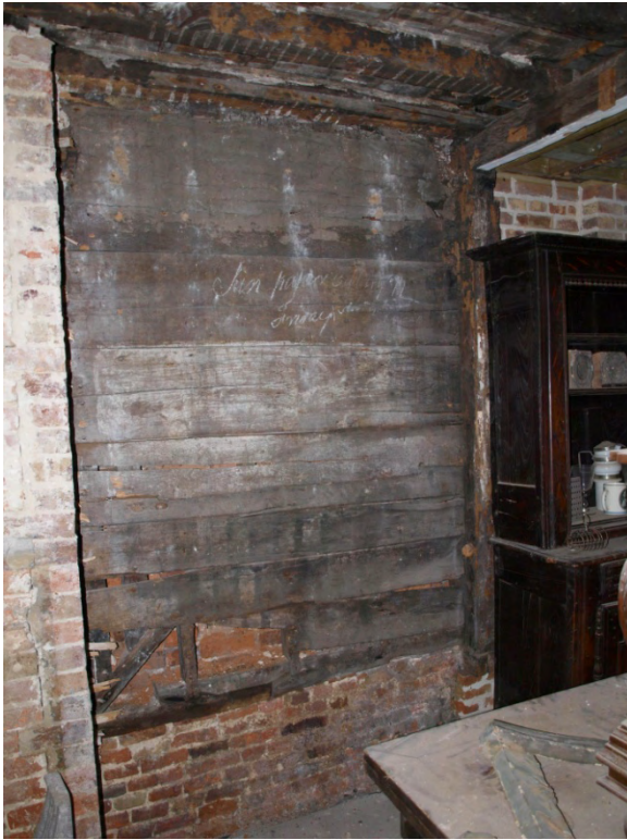
Plate 5: Main range – detail of the boarded northeast end wall, shows studs and straight raking shore jointed to sill beam over earlier brick sleeper wall
