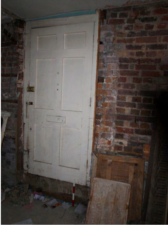
Plate 1: Main range - interior detail of the front door in the principal (northwestern) elevation (400 mm scale)
