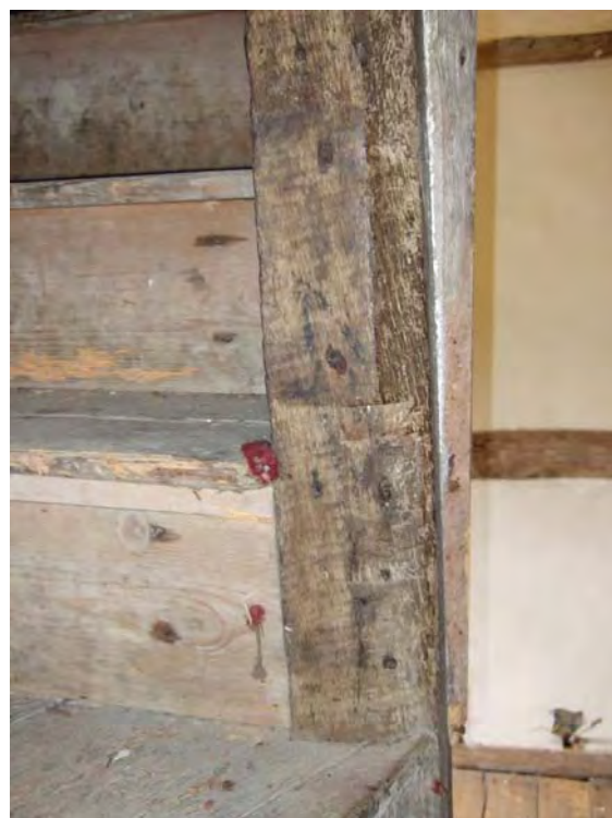
Plate 4 Redundant notch for former winder.
