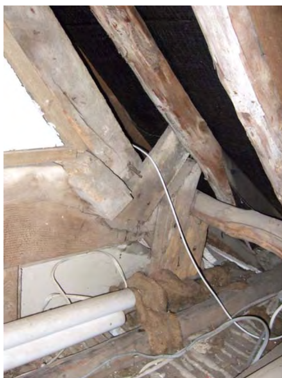
Plate 8 Whitened pole rafters within addition of c.1800, looking south towards period-A northern end wall. Note shallower pitch of rear slope to added roof
