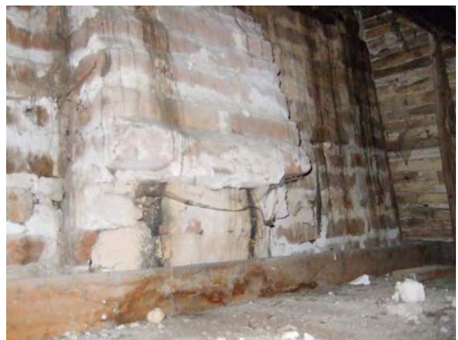
Plate 3 Cut-back remains of tumbling to former flue serving service outshut, viewed from north.
