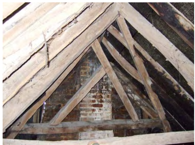
Plate 5 Arrangement of jack rafters above butt purlin within the northern period-D hip.
