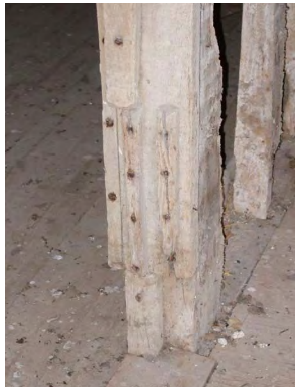
Plate 2 Base of door jamb leading into drying chamber (right). Note slides for lift boards, impression of steps and lath marks on righthand face of studs, terminating at former floor level.
