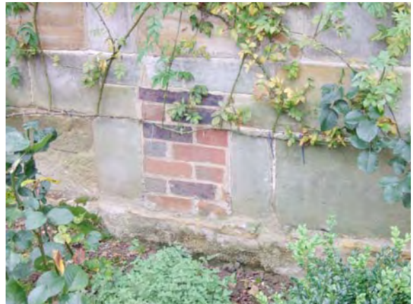
Plate 1 Blocked vent in north wall (others in south wall similar).
