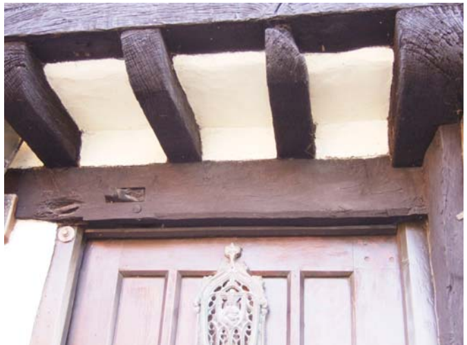
Plate 4 Mortice in jetty plate with hinge pintle to left and chamfered surround to doorway to right.
