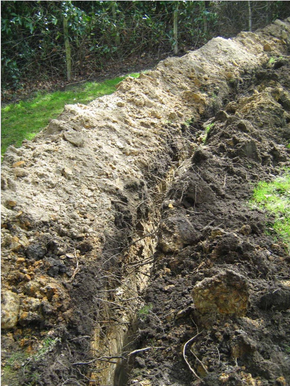
Plate 4: View of cable trench showing the typical sequence of topsoil over clay
