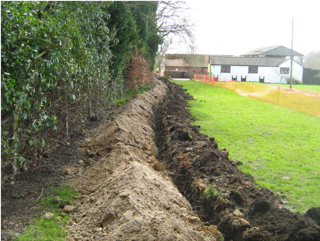
Plate 3: View of cable trench looking south with farm buildings in the distance
