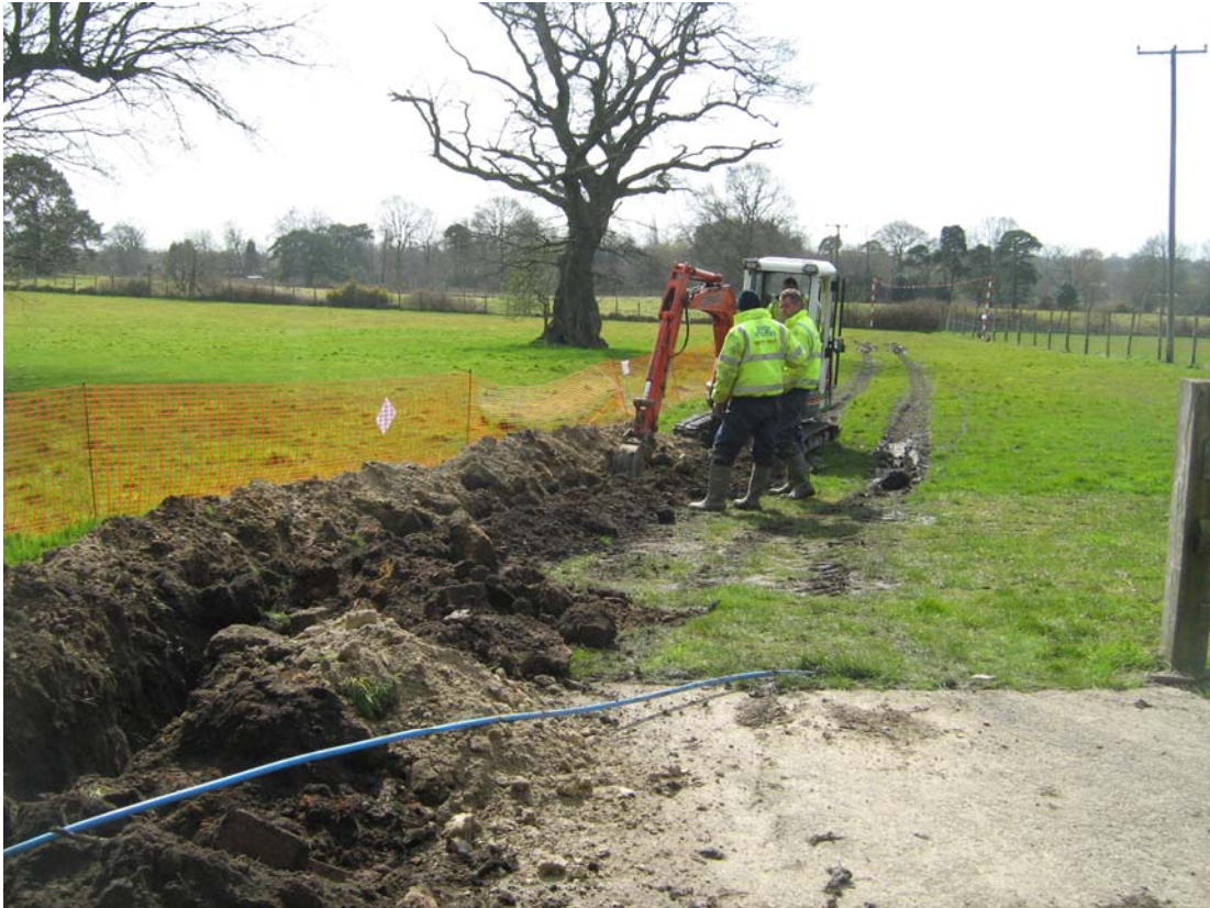
Plate 1: View of cable trench looking south out into the field behind Warley Farm Cottages
