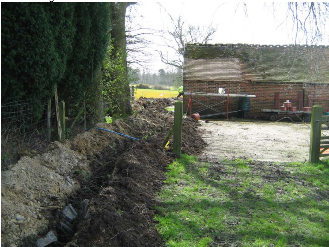
Plate 2: View of cable trench looking south with farm buildings to the west
