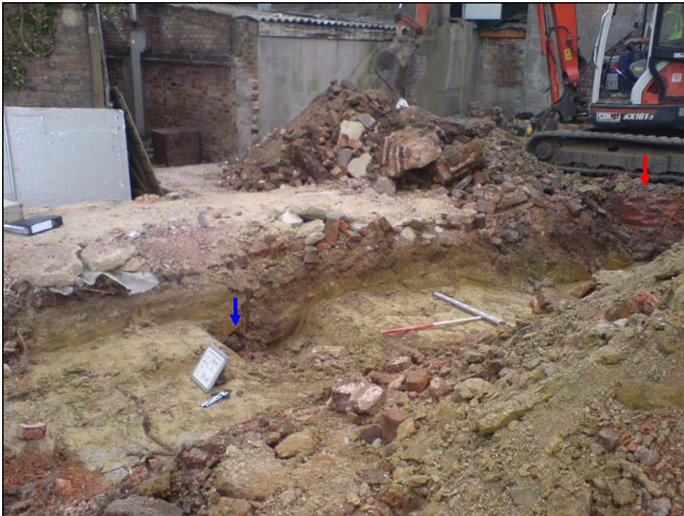
Plate 3: North-west facing shot showing the drain pipe in the side of the trench (blue arrow) and the brick structure at the northern corner (red arrow)
