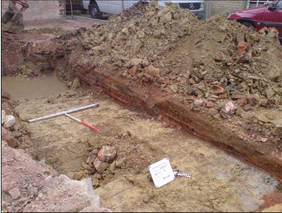
Plate 2: North-east facing shot showing the brick wall running along the south-eastern edge of the trench
