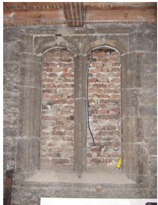
Plate 7 Blocked rear window serving hall
