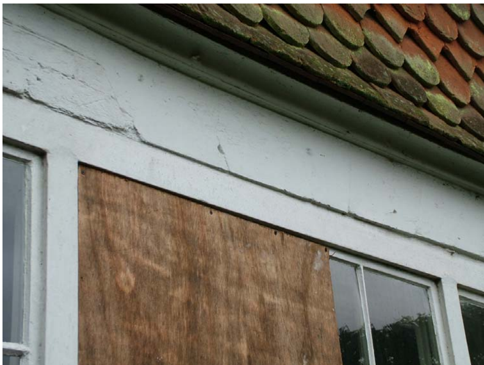
Plate 10 Head of former window exposed above inserted tripartite double-hung sash in front elevation.
