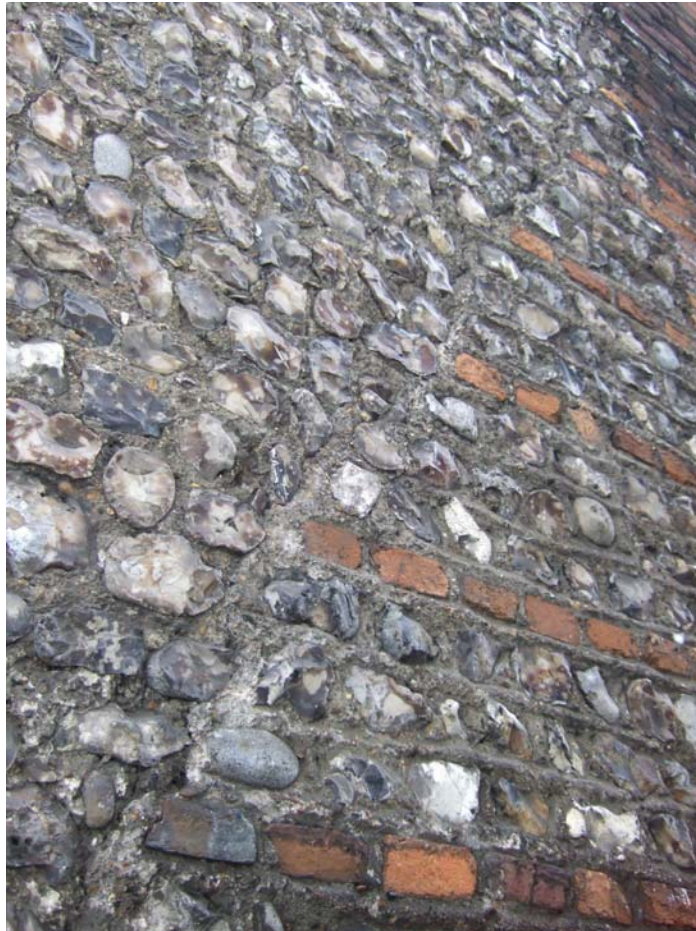
Plate 10 - Scar left by chimney removed from northern wall, with period-B making good (left) incorporating brick banding.
