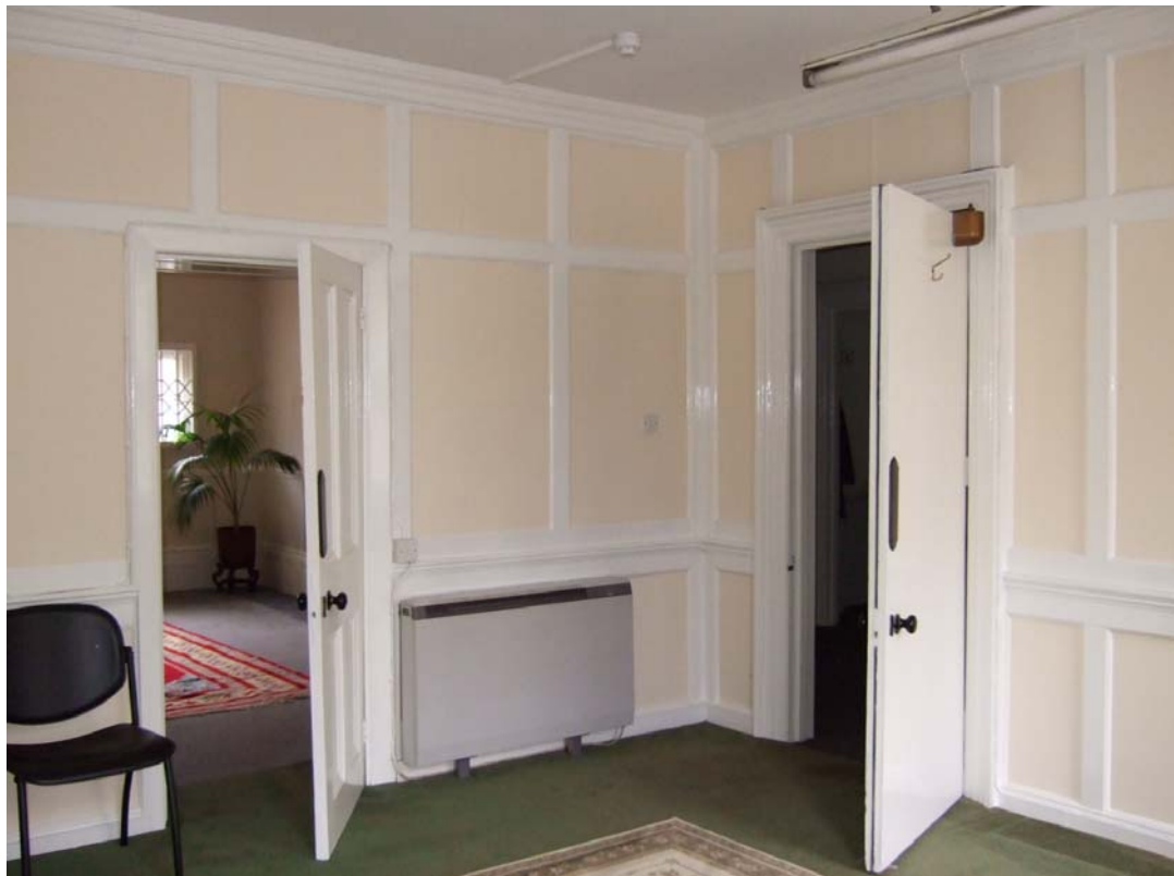
Plate 4 - Panelling in ParLOUR showing intruded doorway (left).
